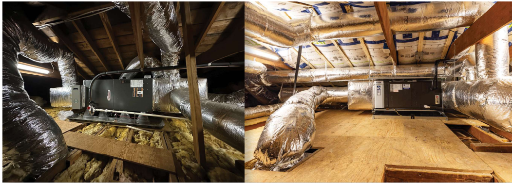
BEFORE | AIR & INSULATION
